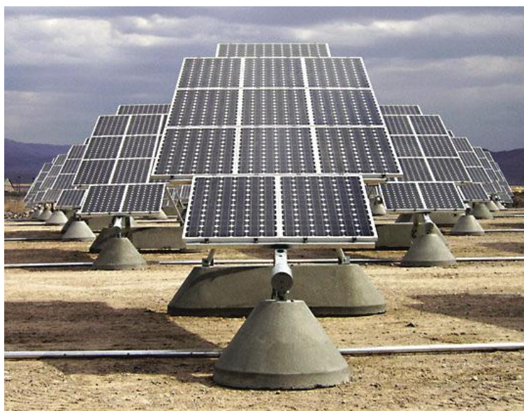
Figure 2. Photovoltaic system with portable crystalline panels with dual-axis tracker
