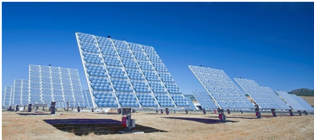
Figure 3. Photovoltaic system with concentrating portable panels with dual-axis tracker Source: from Schwartz (2008)
