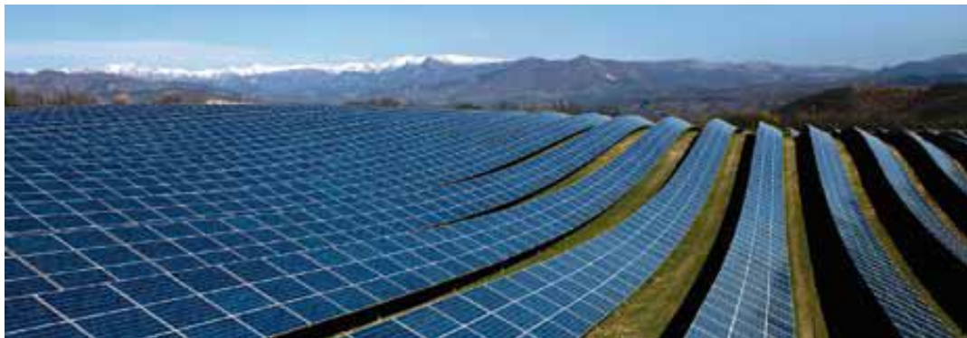
Figure 1. Photovoltaic system with rigid crystalline panels Source: from Remmers et al. (2012, p.11)
